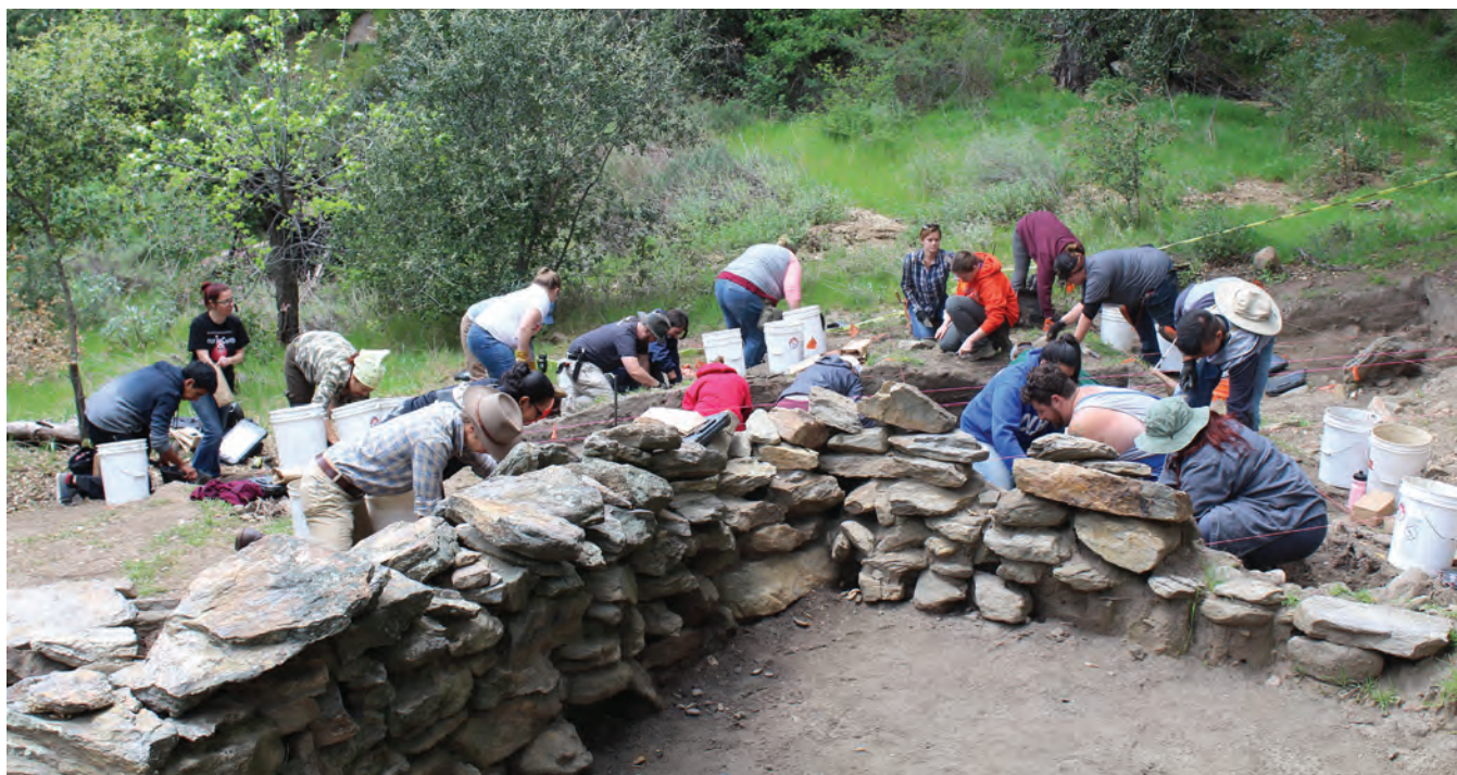
Figure 6.28. The Spring 2017 field crew moved more dirt at the Nate Harrison site than any of the previous field schools; of course, the program enrolled twice as many students as in the 2004-08 excavation seasons.
