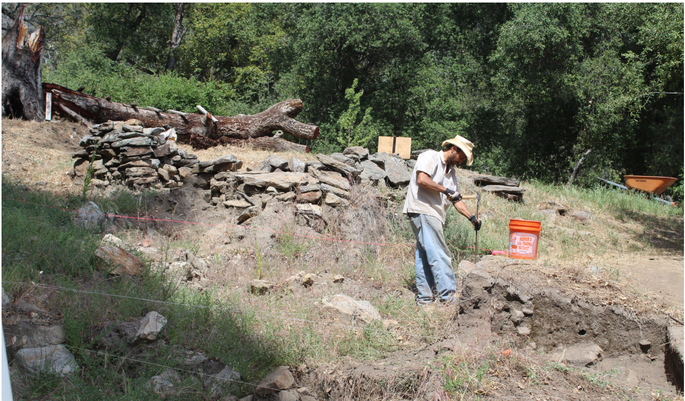
Figure 9.67. Rebar stakes and pink string were used to delineate the backfill area (Courtesy Nathan Harrison Historical Archaeology Project).
